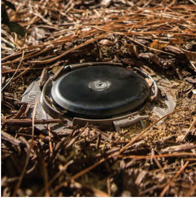
The in-ground housing of the station is secured with a quik-lock cap.
