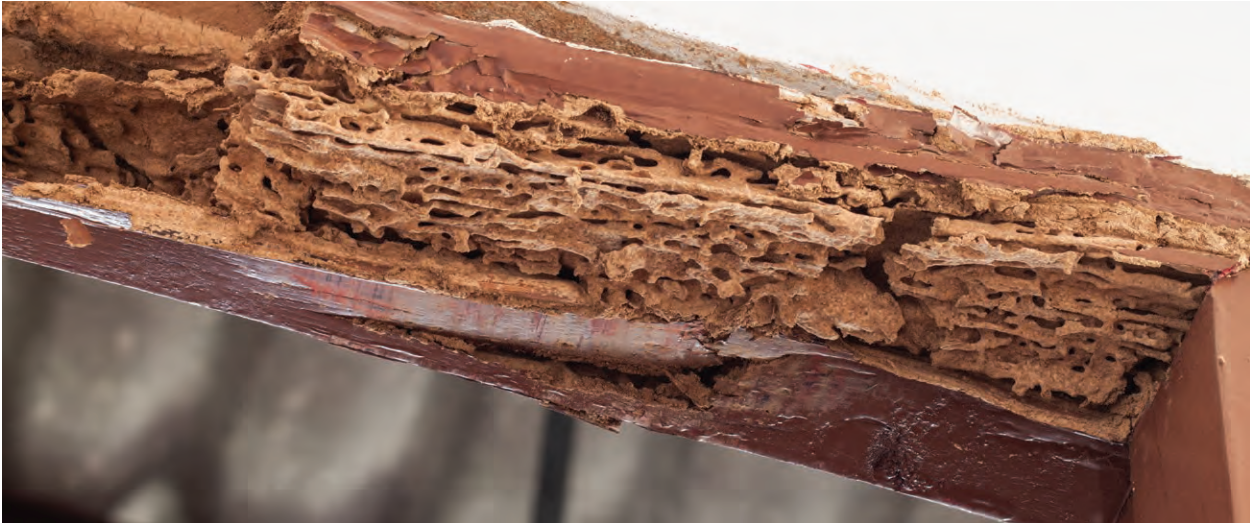
Termite damage to wood
