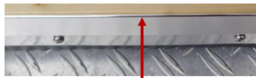
Upper edge of an installed carpet trim of the angled flat bar type
